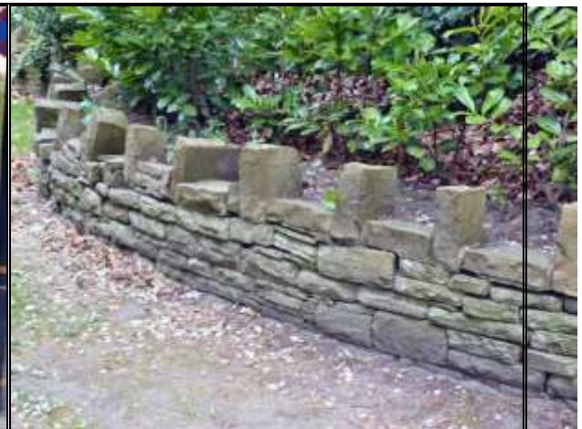
Photograph 103: Low Stone Wall
