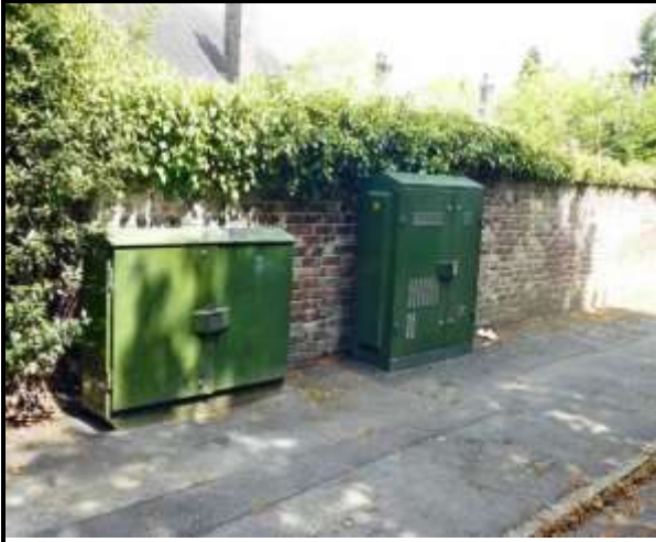
Photograph 26: Services Cabinets, Booth Road
