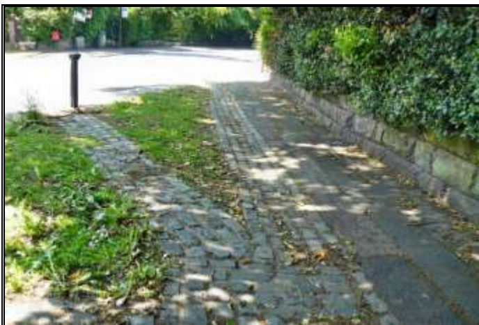
Photograph 78: Areas of setts and Metal Bollards Park Road and Church Brow
