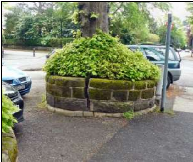
Photograph 117: Cracked Stone Planter, St Margaret's Road
