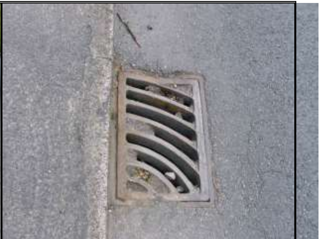
Photograph 99: Drain Cover, Charcoal Road
