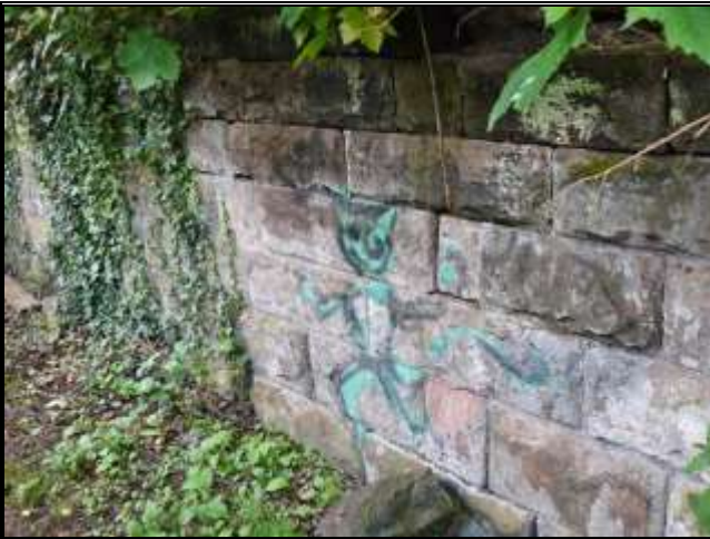
Photograph 129: Graffiti along Passageway in Character Zone A
