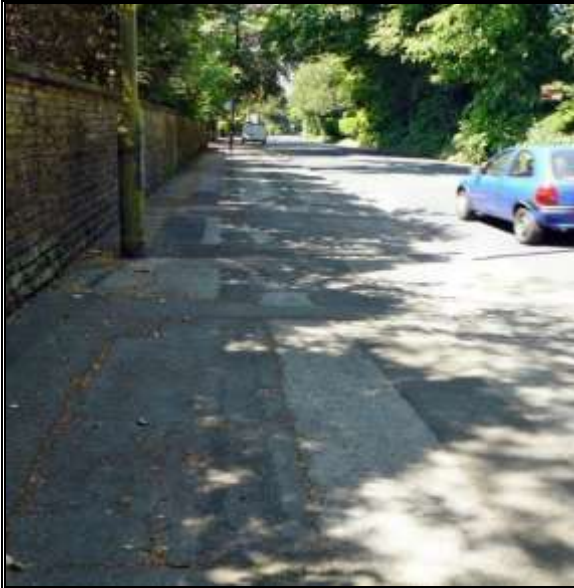
Photograph 127: Example of Patch Repairs, Park Road
