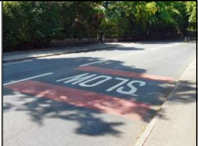
Photograph 126: Inappropriate Road Markings, Park Road
